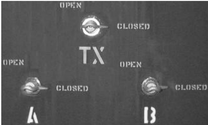
Figure 23. Loop switch with ON-OFF radial switch.
