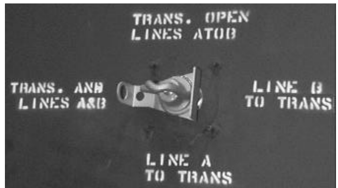
Figure 25. T-blade sectionalizing switch.
